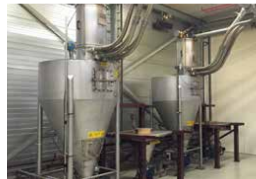
RECEIVING HOPPERS WITH FILTER
