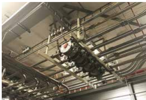
CONVEYING LINE, AIR ASSISTS AND DIVERTERS
