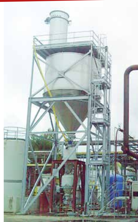
L-I-W dosing system & dense phase conveying
