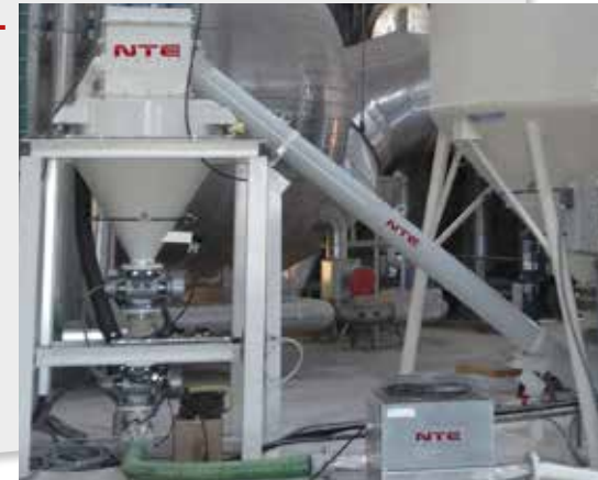
Unit for SO 2 and HCl removal with Eco-Lance®
