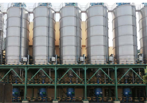
STORAGE SILOS & DENSE PHASE PNEUMATIC CONVEYING
